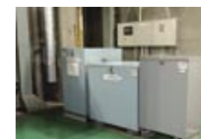
PCB storage EnoKicho Plant, Commercial Printing Operations
